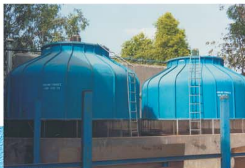
Two numbers of cooling towers having a total capacity of 1200 TR.
